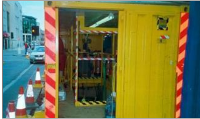
Figure 12 - HV cable jointing container
